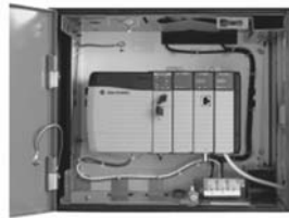
Programmable logic controller (PLC)
